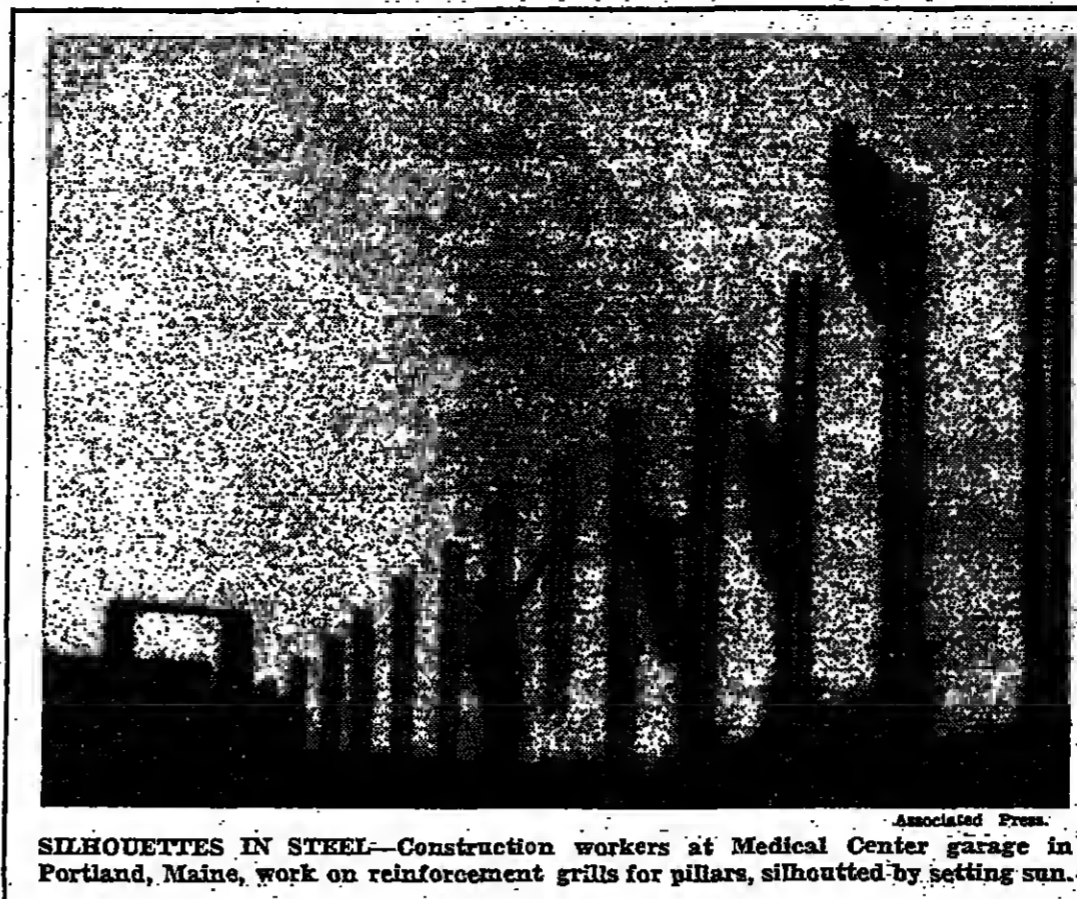
SILHOUETTES IN STEEL—Construction workers at Medical Center garage in Portland, Maine, work on reinforcement grills for pillars, silhouetted by setting sun.
